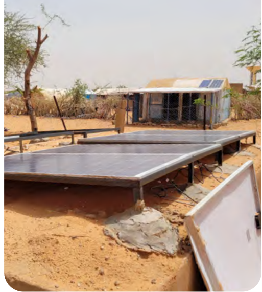
Solar panels in need of maintenance
